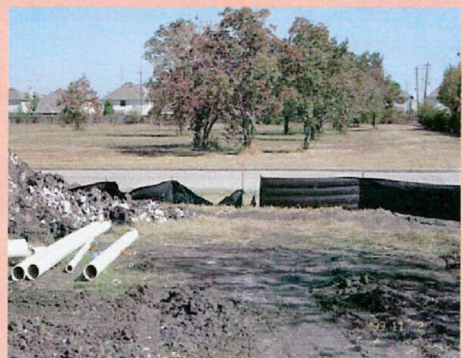
Poorly Maintained BMPs MPGs Pobremente Mantenidas
